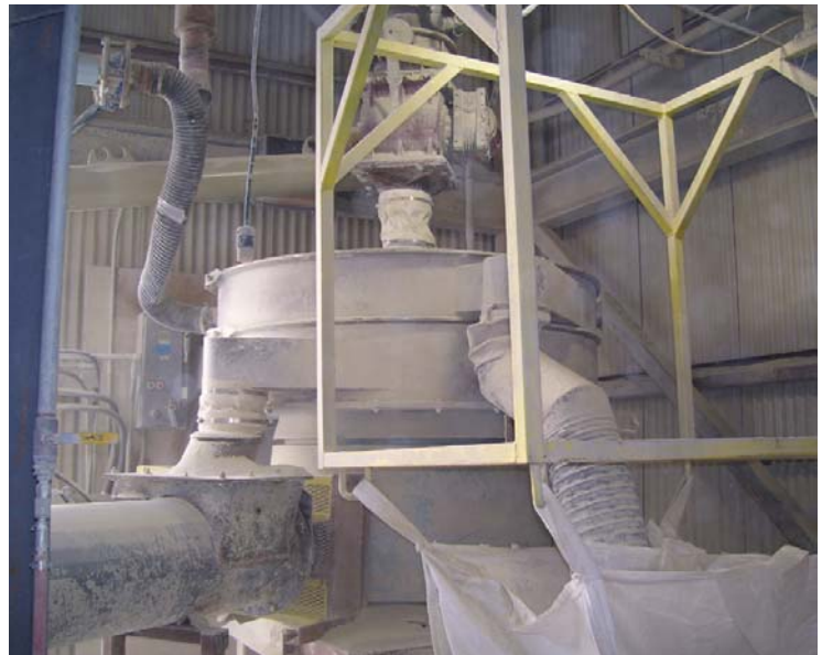
A Russell Finex separator in use at Zemex's plant
